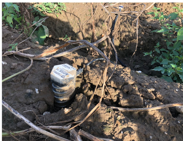
Figure A1. Picture of a SoilVUE10 sensor in the Leerodt field showing loss of soil contact due to soil erosion.
